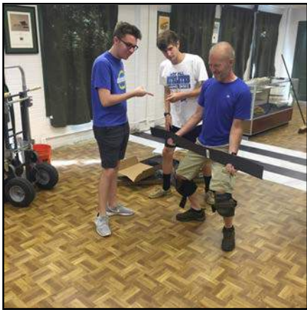
Museum members John William and Andrew Davis put the finishing touches on the floor of the community room/Ready Room for Andrew's Eagle Scout project.
